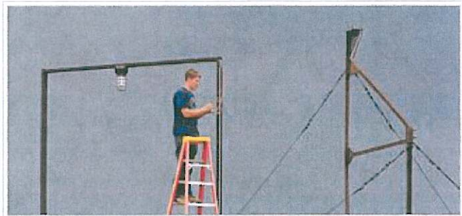
Kyle Osborn works on wiring the overhead lights on the Garfield Street pedestrian bridge. Andy Carpenean/Boomerang photographer
