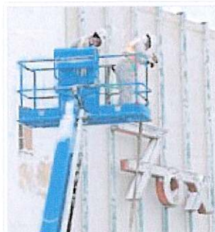
Workers wearing protective gear hover Monday above the old Fox Theater during work to collapse the theater's decaying roof. Andy Carpenean/Boomerang photographer
